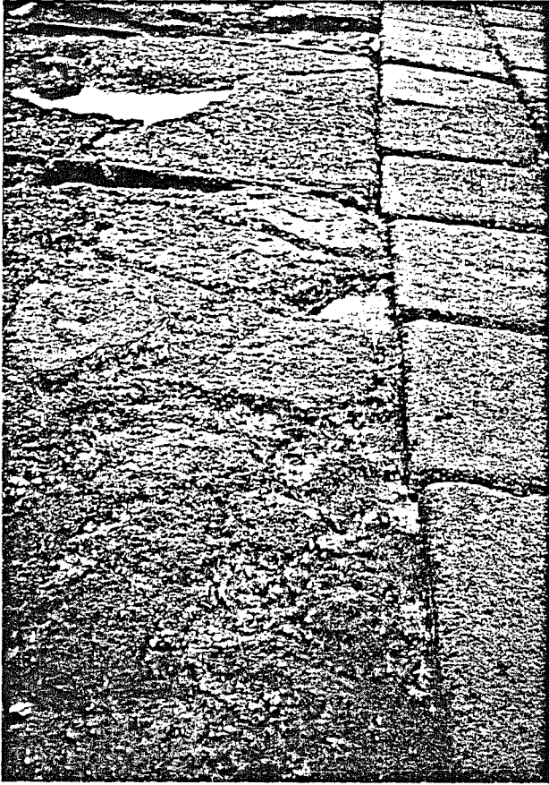
Poor and good concrete side by side.
