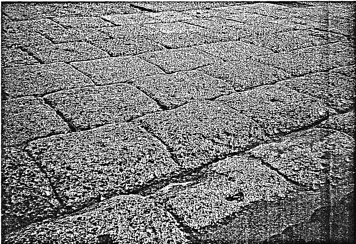
Severe erosion due to the scouring action of granular material and water.
