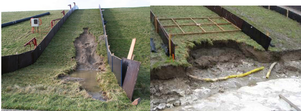
Figure 3.2 Geometrical transitions (at toe of dike), on the left: Boonweg, on the right: Kattendijk
