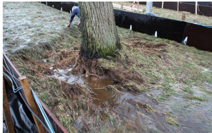
Figure 3.3 Erosion at tree (halfway the inner slope of the dike)
