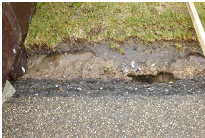
Figure 3.1b Multiple open spots at transition from asphalt road to grass revetment (after 12h at the end of q = 10 \ell/s per m)
