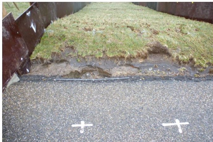
Figure 3.1c Failure of transition from asphalt road to grass revetment (after 14 h or after 2h with q = 50 \ell/s per m)
