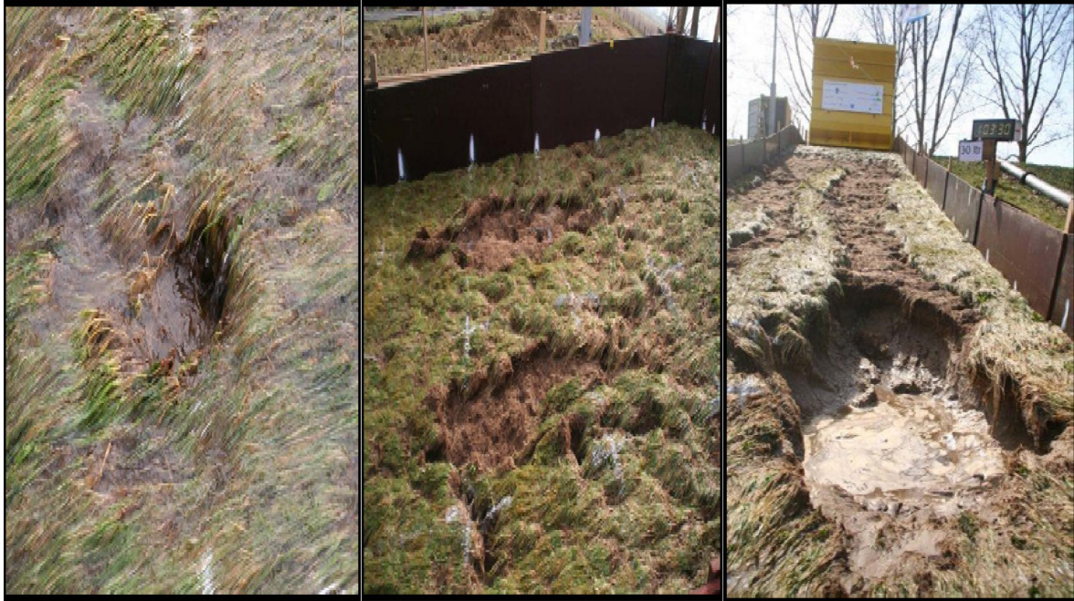
Figure 2.1 Initial damage, damage at multiple locations and failure of embankment
