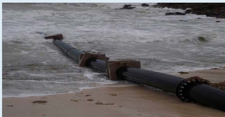
APUA RO intake line: concrete anchors shifted and line displaced.
