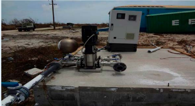
Barbuda Reverse Osmosis (RO) plant: pump station completely destroyed, transformer overturned and roof of the plant damaged.
