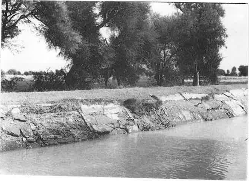
Figure 4C. Damaged Lining of Mohajar Branch.
