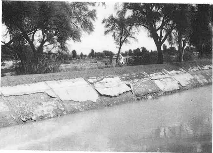
Figure 4D. Damage to Plaster Used to Repair Lining Mohajar Branch.
