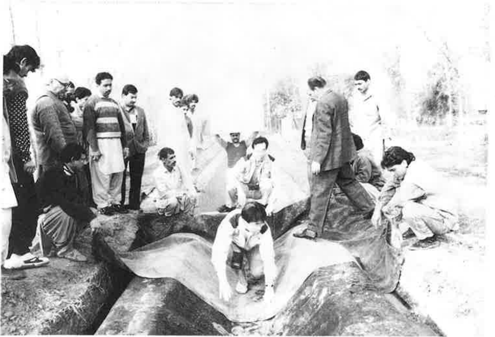
Photo 11. A view of providing extra sheet piece at end points in lined section to avoid bond problem at Niaz Beg Research Station, Lahore.
