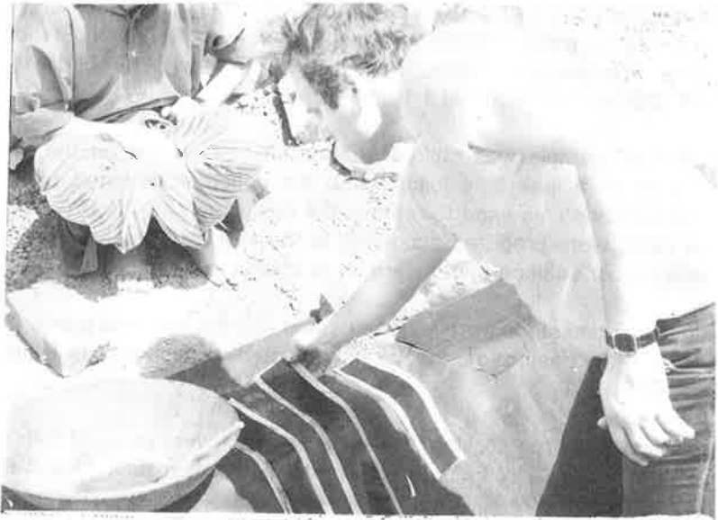
Photo 4. Butyl adhesive strips prepared prior to joining the Taurus rubber sheet with pillars Niaz Beg Research Station, Lahore.
