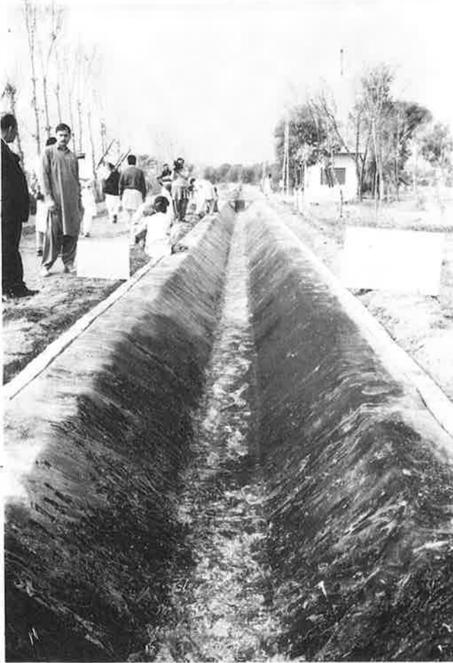
Photo 10. Mizu rubber sheet installed in exposed condition in water channel section at Niaz Beg Research Station, Lahore.
