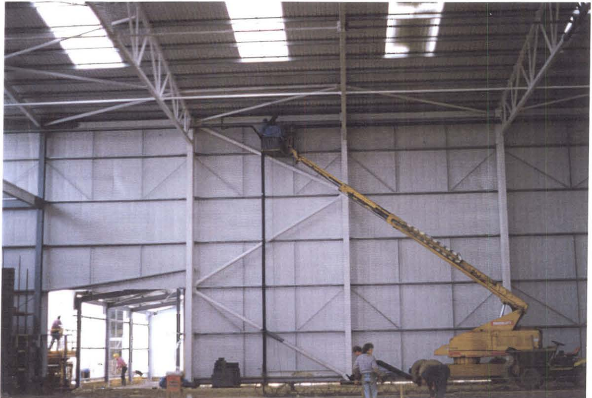
Plate 1 Installation of siphonic system in a building
