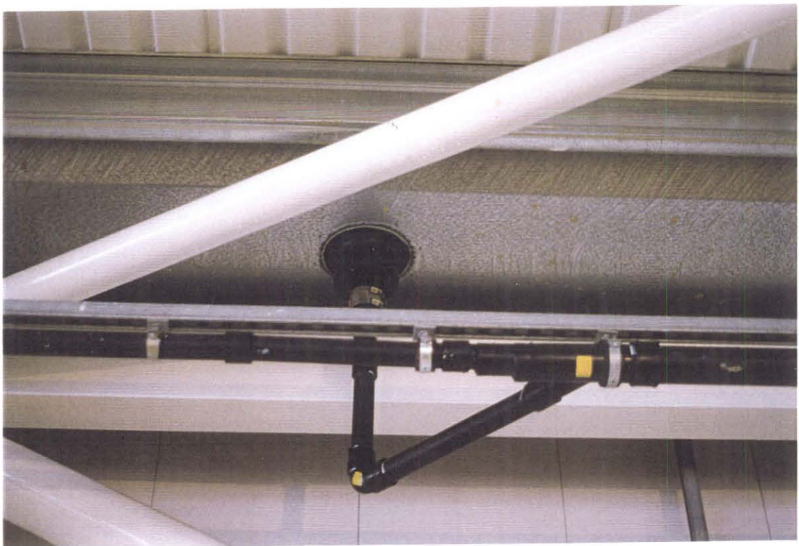
Plate 2 Tailpipe connecting outlet to a collector pipe
