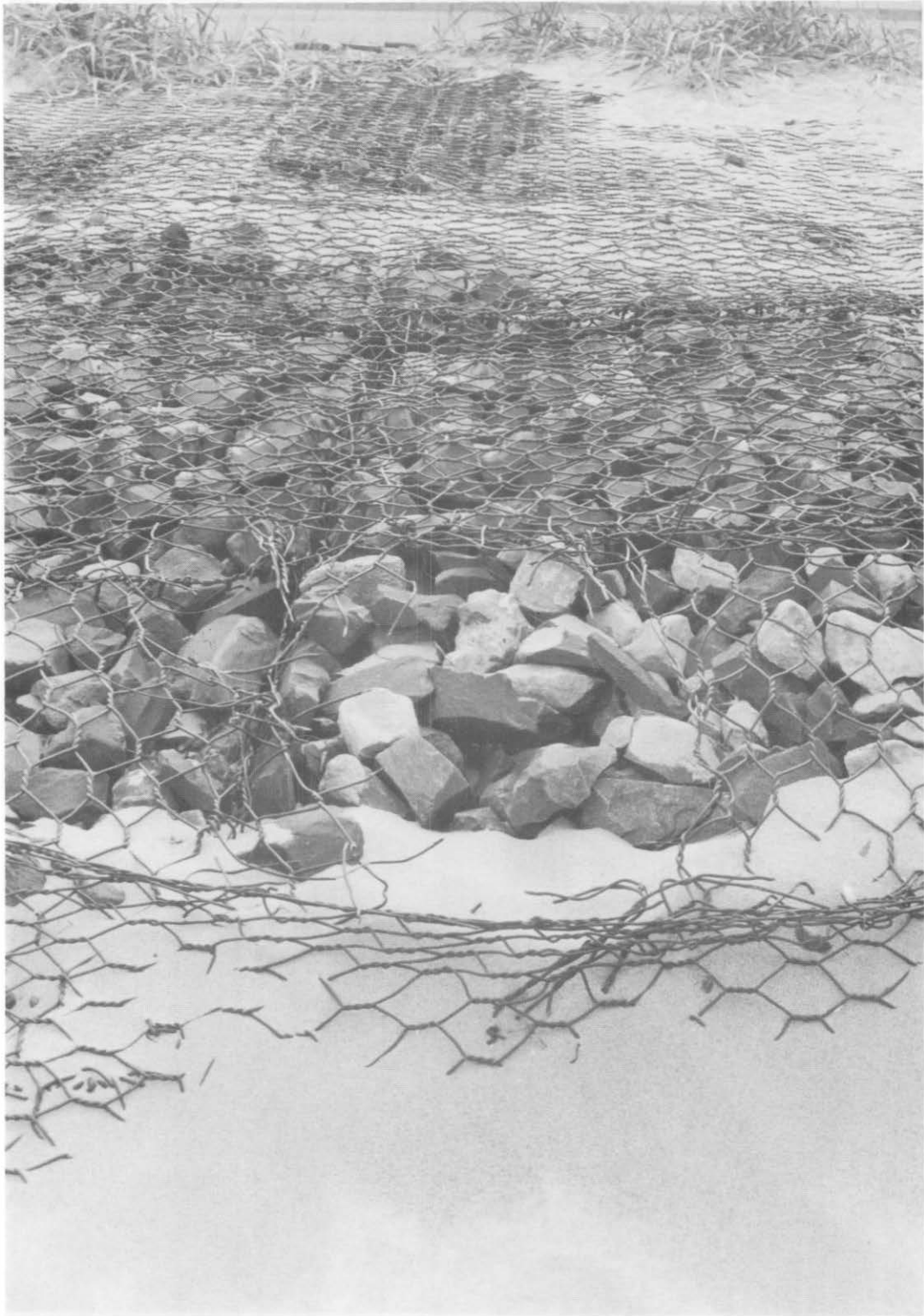
Plate 15 Example of damaged gabion revetment
