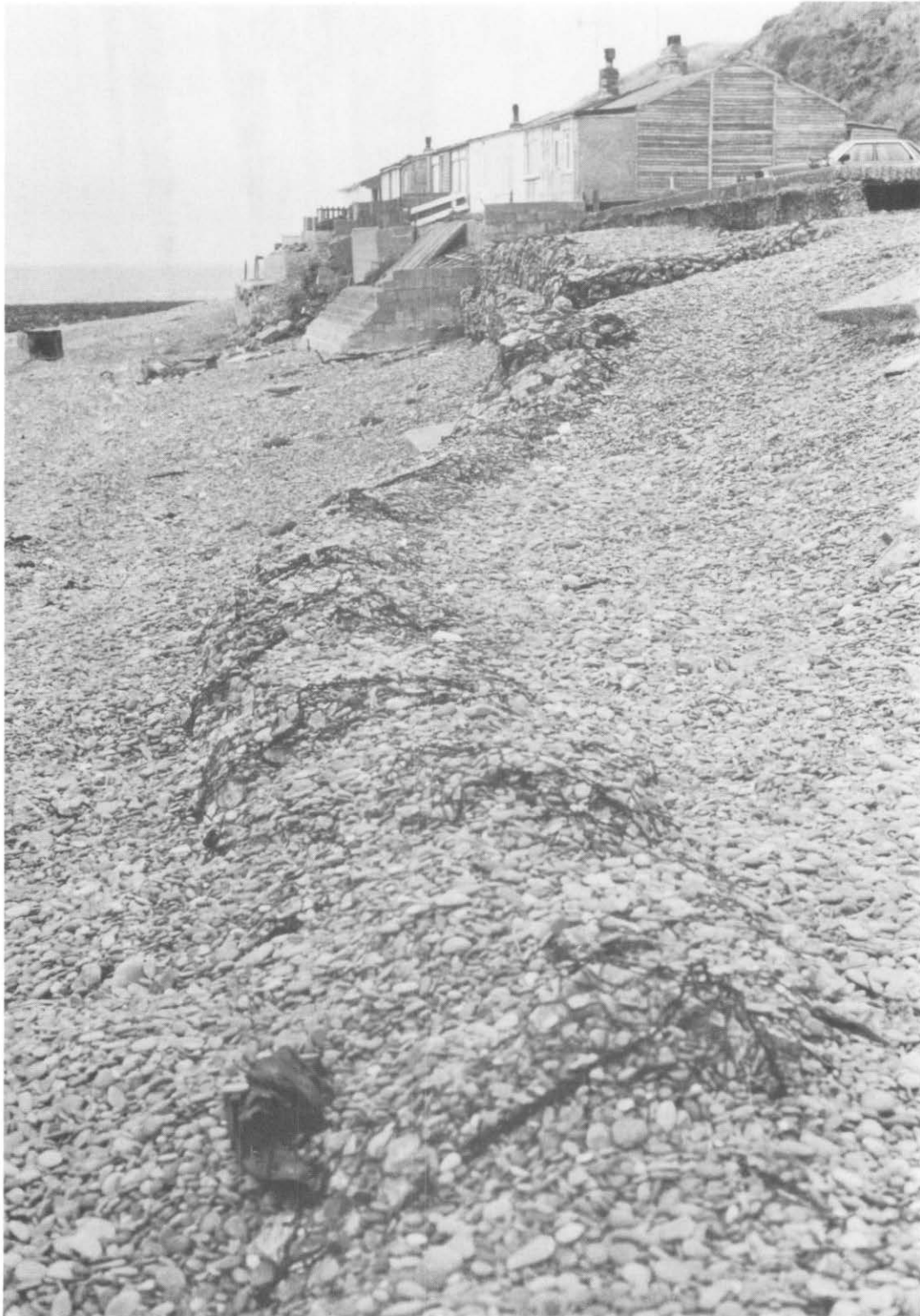
Plate 13 Damaged sea wall on shingle beach
