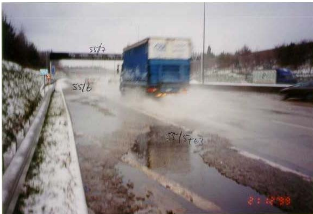
Plate 2 Ponding on M25 (Route A) between Junctions 8 and 9 due to lack of camber
