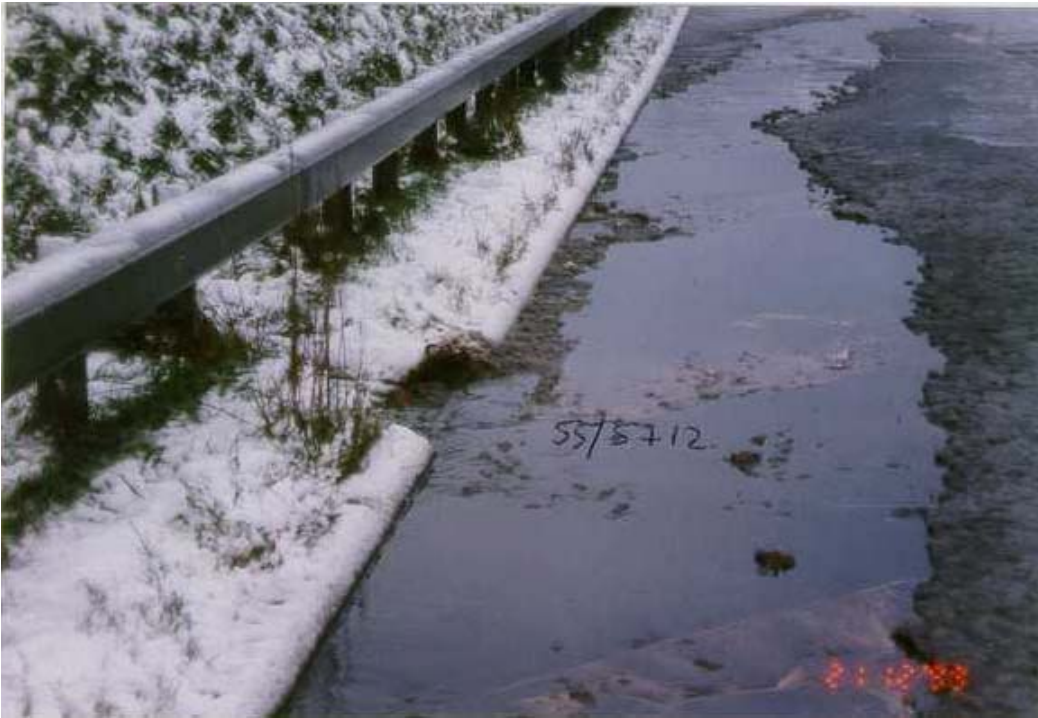
Plate 3 Flow by-passing recessed gully on M25 (Route A) between Junctions 8 and 9
