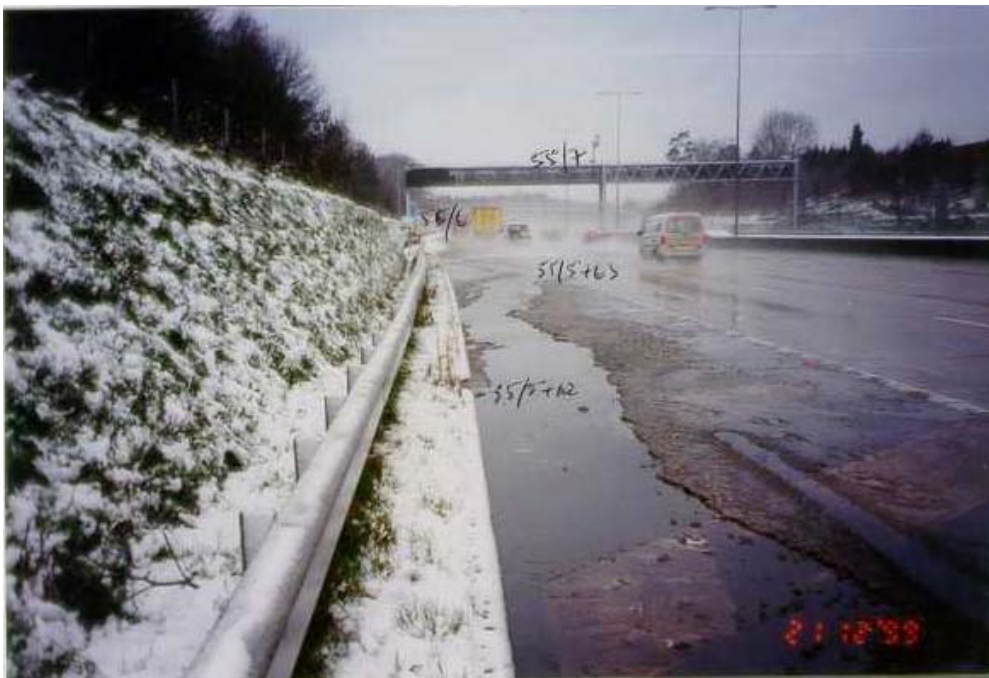
Plate 6 Ponding on M25 (Route A) between Junctions 8 and 9 due to lack of camber
