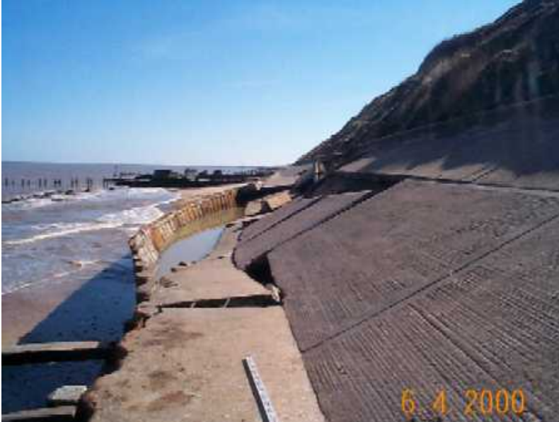
Figure 2: Seawall damage on the east coast of England (photograph courtesy of Waveney District Council)
